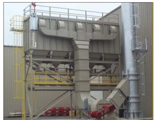
405MBT8 at brick manufacturing facility
