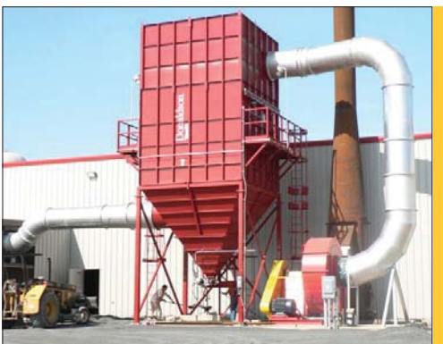
324MBWS10 at a glass manufacturing facility
